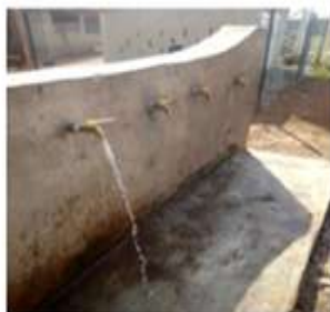
Plate 1 C: Kere-aje motorized borehole
